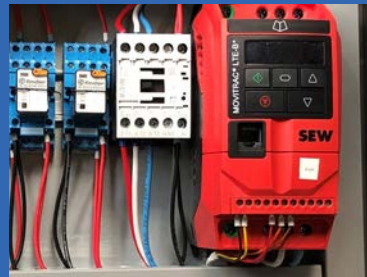
Variable Speed Drive
