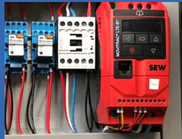
Variable Speed Drive
