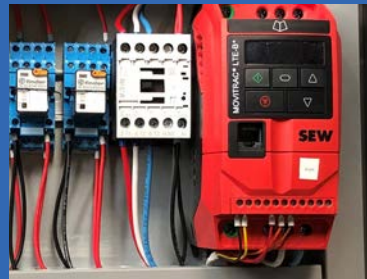
Variable Speed Drive
